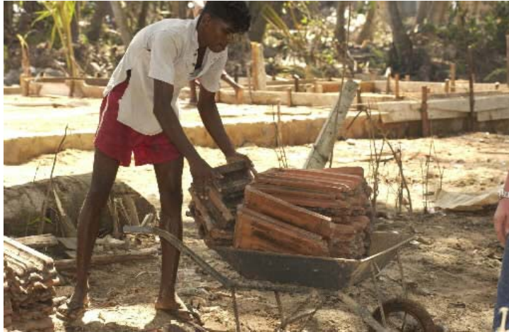
Building is under way in Galle for families who have title to their land. Habitat is providing some of the raw materials and skilled masons. Other materials include debris gathered by homeowner families and volunteers.
